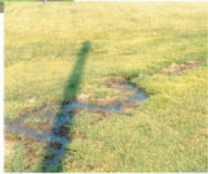
Surface discharge from non-compliant septic system that would be considered an imminent threat to public health or safety
