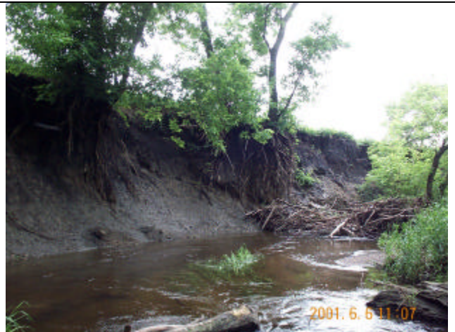
Photo12. Stream bank erosion site.
